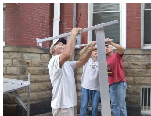
Duane Buck, John Hartigan and Matthew Cornett at work to reassemble the ramp.
