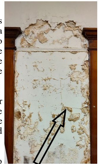
Crumbling wall that will be replaced.
